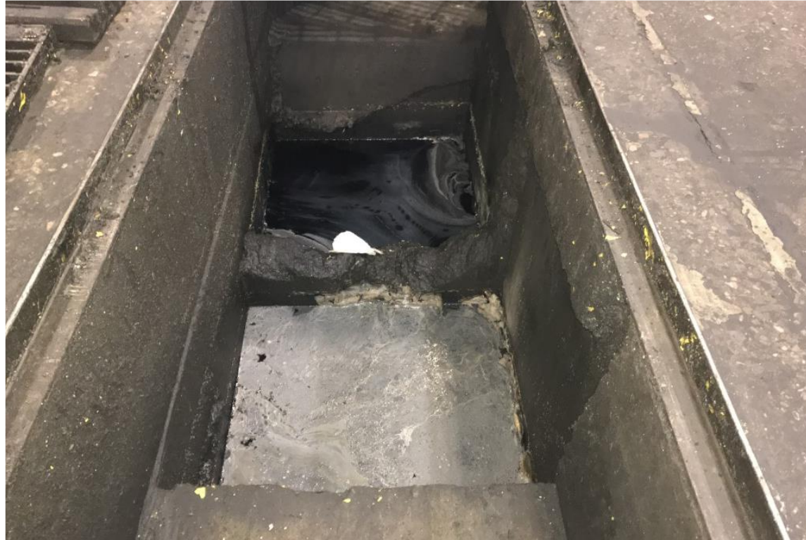
View of a damaged OWS
