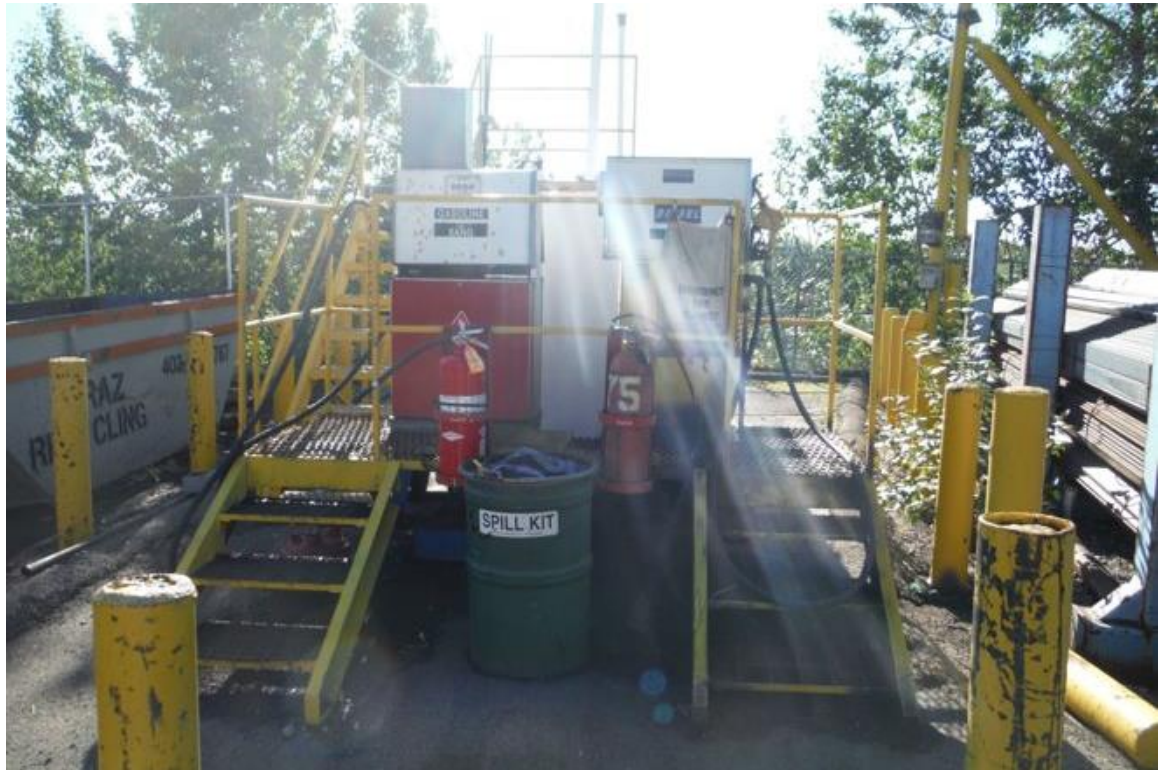
Aboveground fuel storage tank operating without secondary containment
