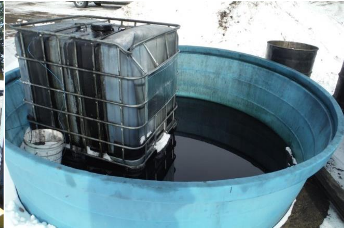
Waste oil storage tote with uncovered secondary containment
