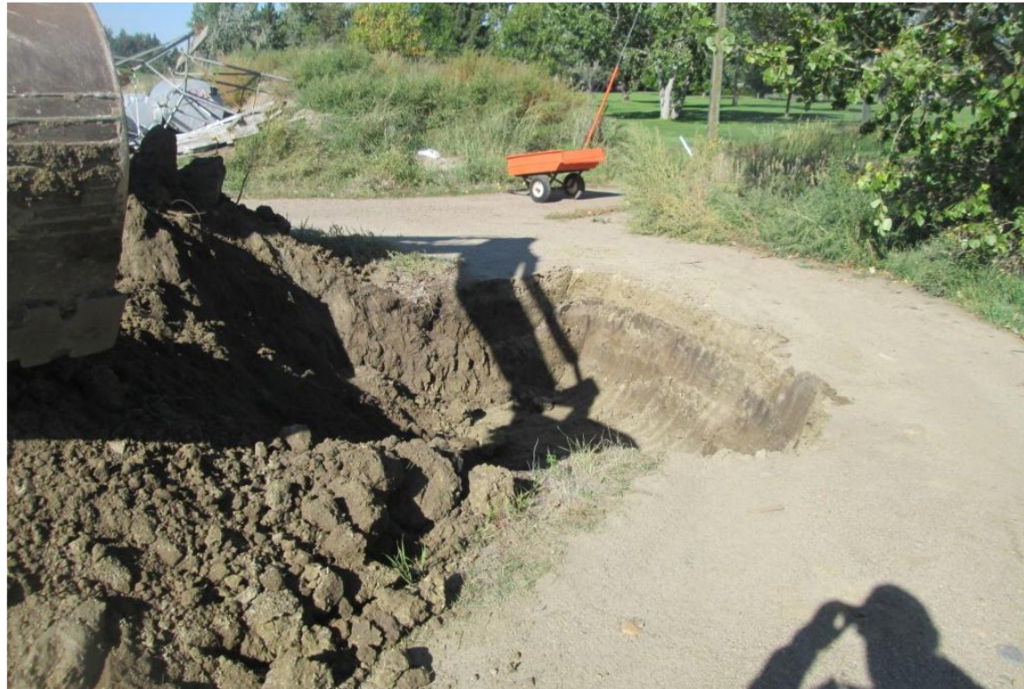
Exploratory excavation of ground around damaged fuel storage tank
