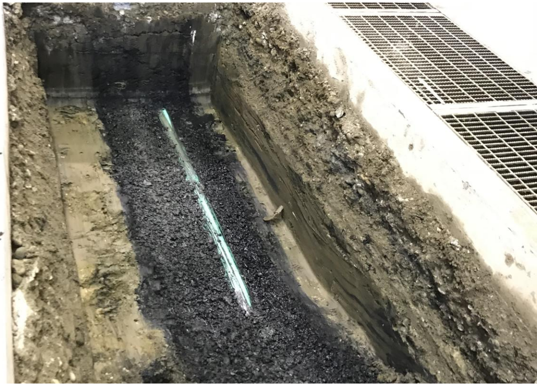
View of exposed contamination migrating through gravel fill material
