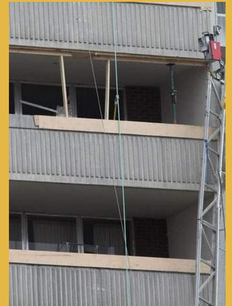
Metron Dec 24th , 2009 Scaffold Issue
